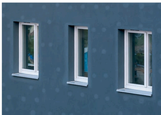
Façade without caps installed to insulate the mechanical fastener plates.
